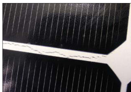
▲ Obr. 3 ● Popraskaná fólie TPT
