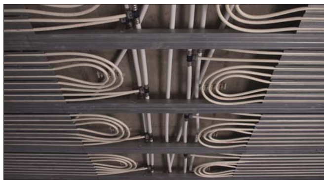
▲ Obr. 1 ● Instalace Wavin Tempower CD-4
